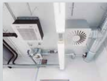
Noise generated by HVAC systems
